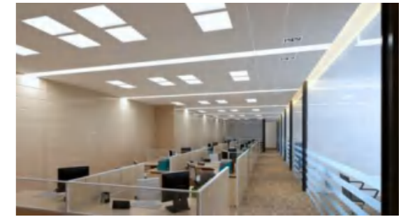
General Lighting for Commercial and Office Spaces
